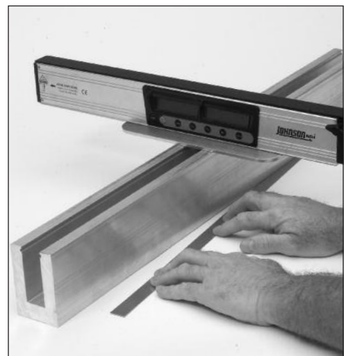
Use the "PAL" Tool to assure the Base Shoe is level at all points
